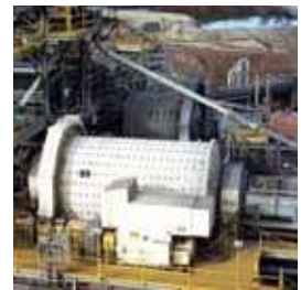
Above top: Metal cap shell plates and lifters plus metal cap lifters on the grate discharge mill end
